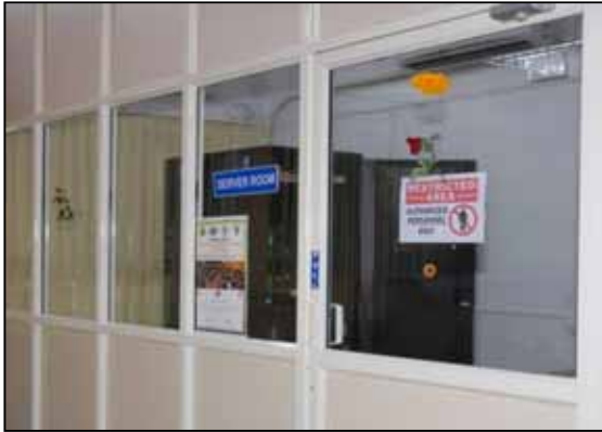
Server Room in order to store and access the data of RFID, Koha and other softwares
