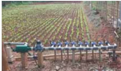
IoT pump controller
