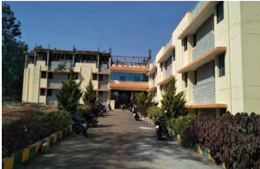
Construction of PG boys hostel 1 st floor is completed & construction of PG boys hostel 2 nd floor is under progress
