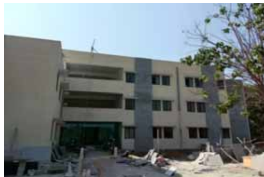
Construction of boys hostel 1 st floor for diploma college at College of Agriculture,V.C. Farm, Mandya is under progress
